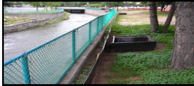
▲ Above: One form of erosion and sediment control practices used on Market Street in Auburn, NY.
