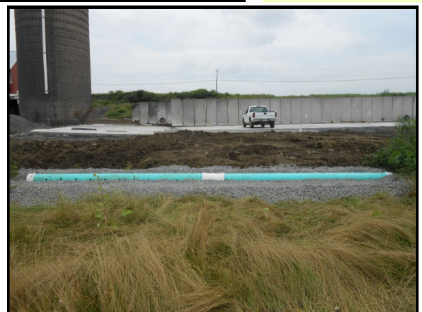
To the right: Level lip spreader distributes dilute runoff across the top of the VTA.
